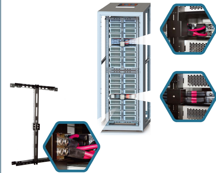
Custom Bus Bar Connection
